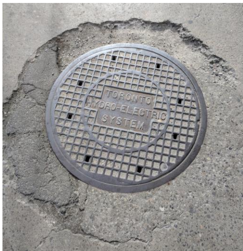
Toronto Hydro-electric system man-hole Source: 4D Infrastructure
